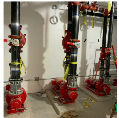
Clean out any pump suction diffusers and equipment strainers.
